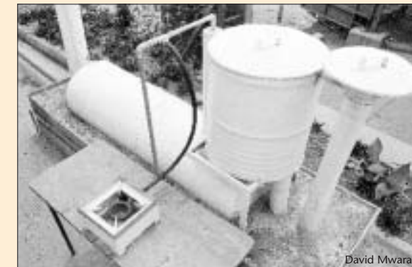
David Mwarira Biogas demonstration plant
