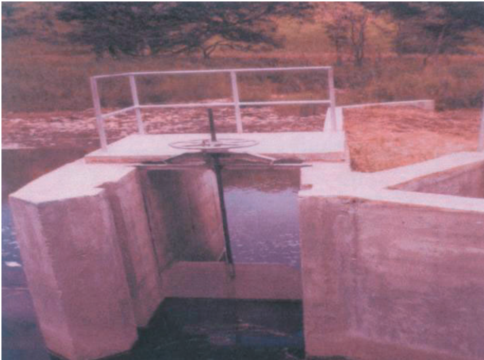
Photo 4.2: Intake of Luanda-Majenje Improved Irrigation Scheme
